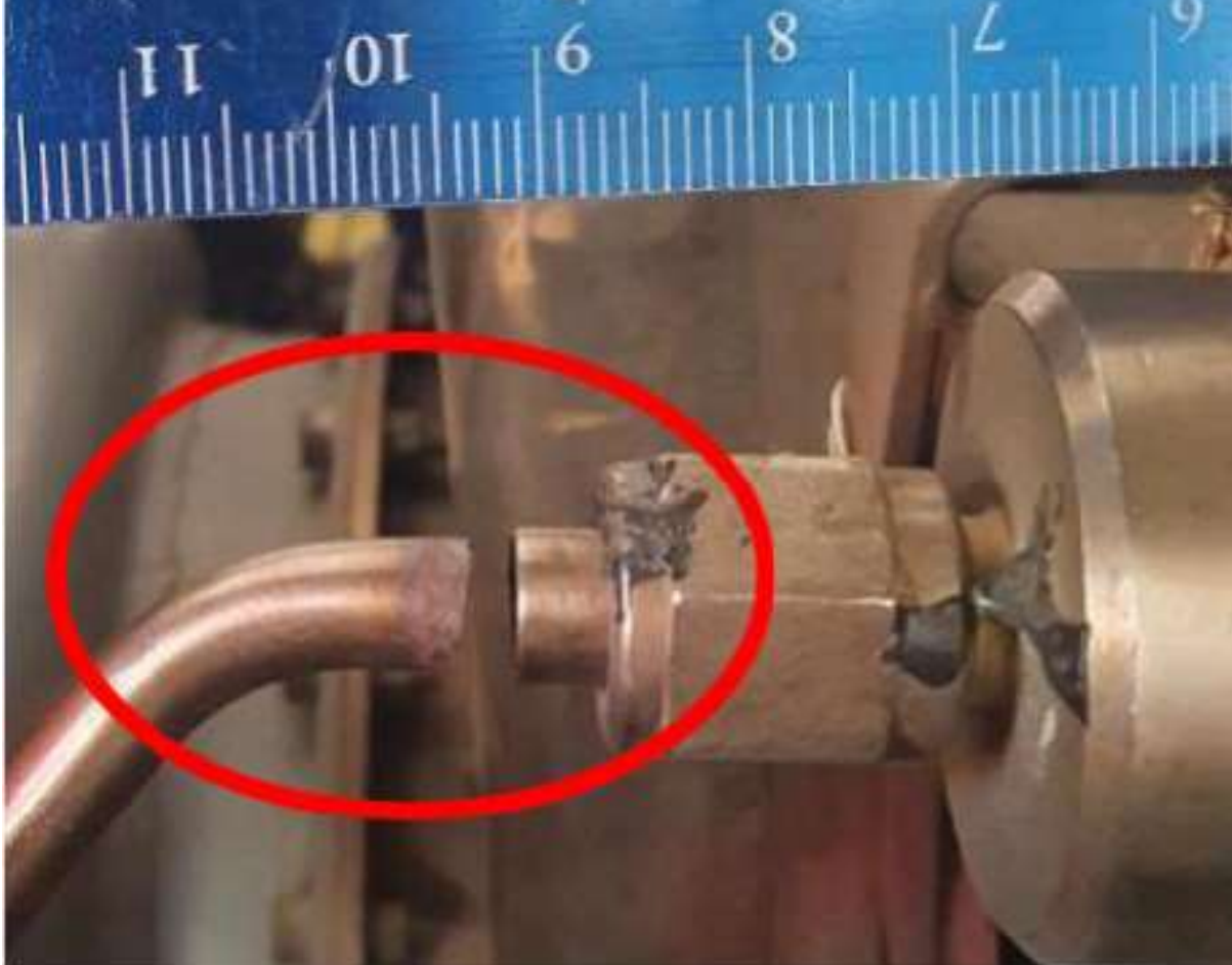
Broken Tubing with Gap Indicative of Misalignment FIG. 11
