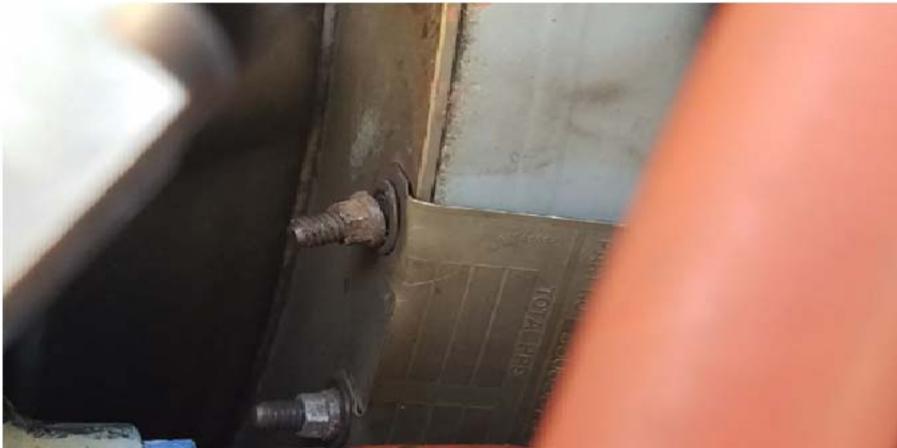
Example of Broken Compressor Diffuser Stud Figure 2
