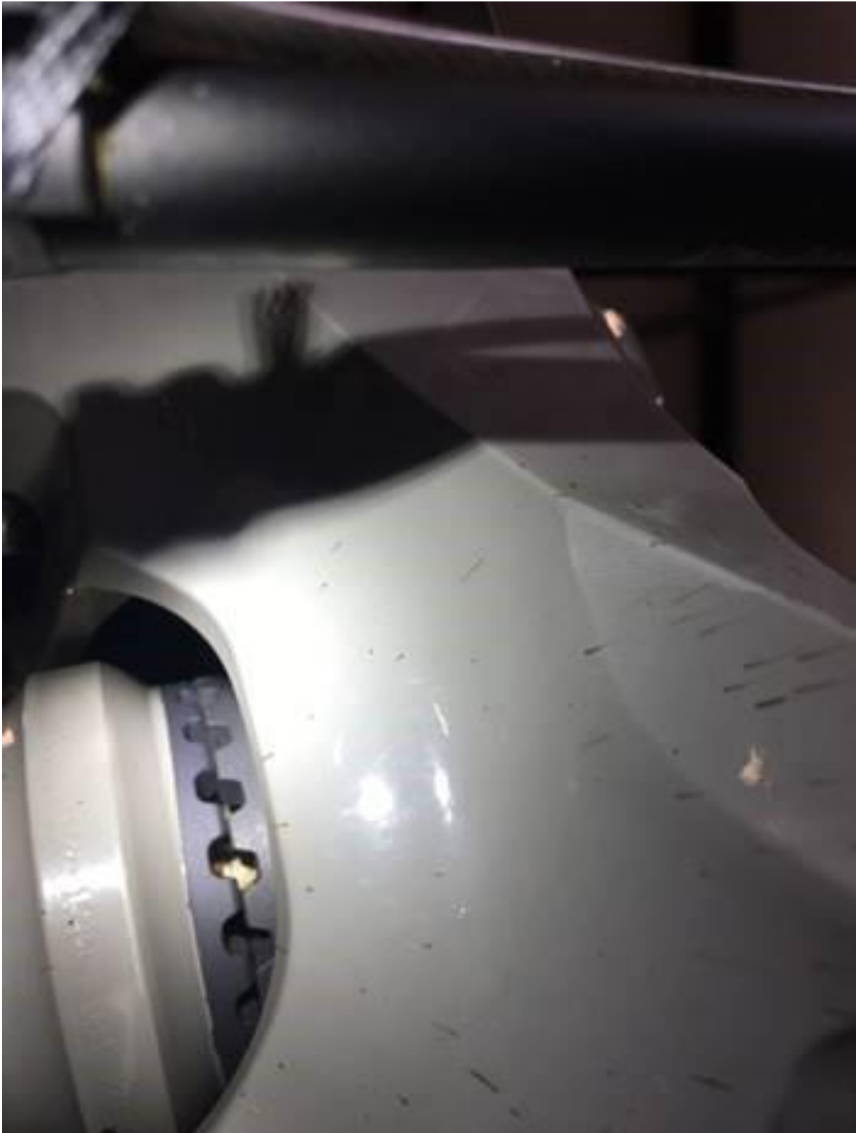
Figure 1 – Example of Improperly Engaged Curvic Coupling
