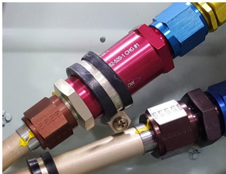
Detail B. Engine Oil Check valve not Manufactured by Circor Aerospace
